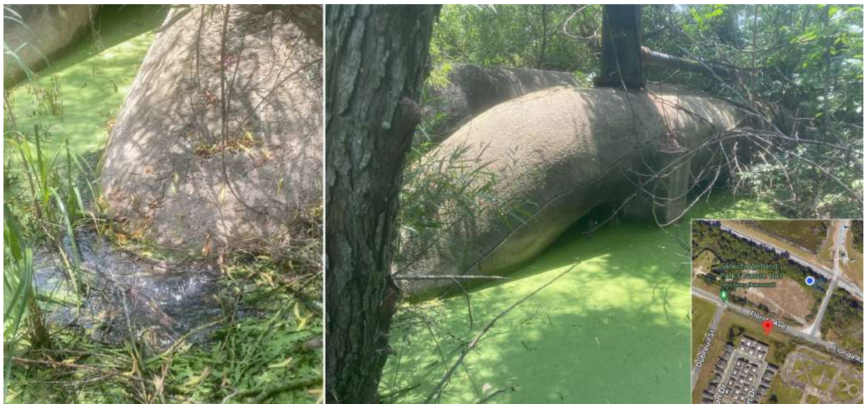
Figure 2. Septic water leakage at the base of the forced main septic pipe leading to the Veolia WTP. The location is indicated by the blue dot in the lower right panel.
